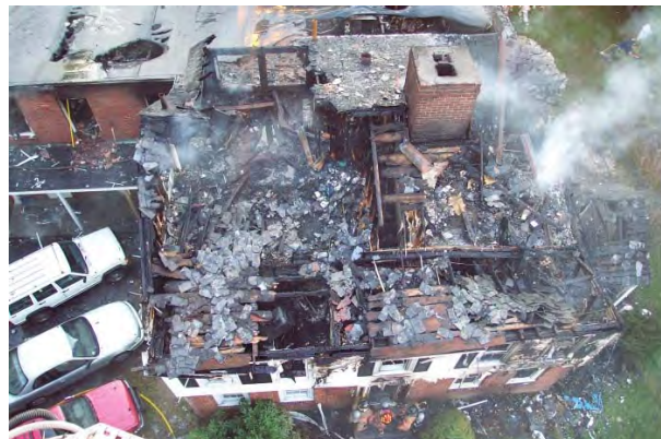
Damage to a college fraternity house, caused by an electrical fire.
